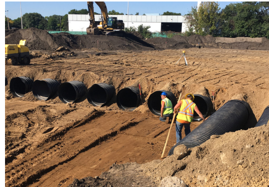
Underground stormwater management
